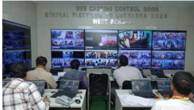
Control room, West Bengal
